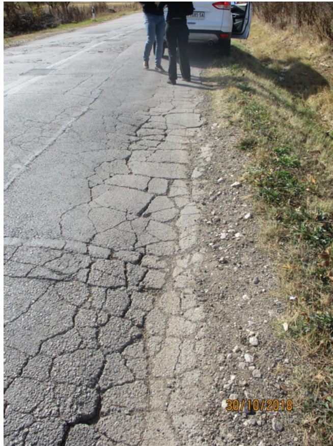
Picture 5. Example of damage
