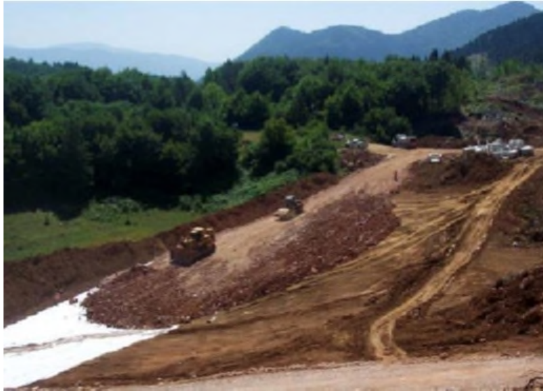
Figure 3-46. Example of Replacing of Embankment Formation (Foundation) with Geotextile and Suitable Material
